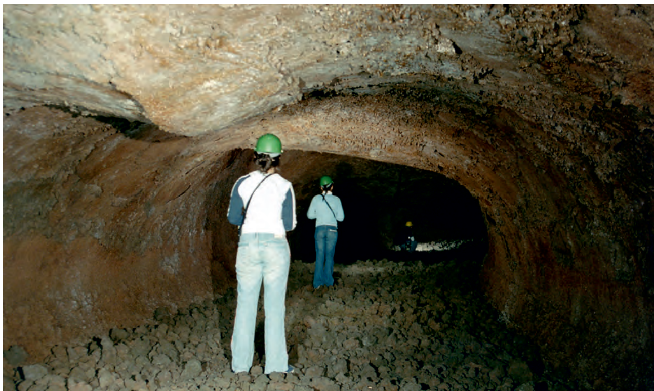
Fig. 9 - Volta del tunnel deformata per collasso, in alto a sinistra (Grotta Cassone). - Ceiling of a tunnel deformed by a collapse, up on the left corner (Cassone Cave).
